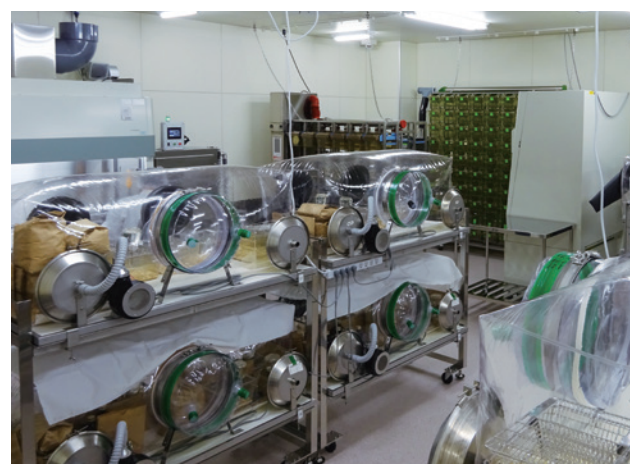
Figure: Vinyl isolators and two types of Individually Vented Cage systems in the new SPF animal facility
